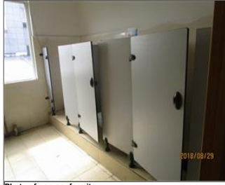
Photo of non-conformity NC-7.22 Restroom without privacy door.JPG
