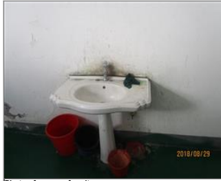
Photo of non-conformity NC-7.22 Hand-wash station without cleaning supply.JPG
