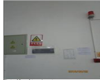
Photo of fire safety equipment Fire alarm device.JPG
