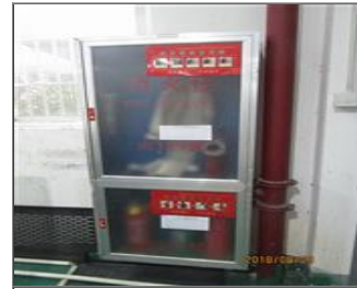
Photo of fire safety equipment Fire equipment.JPG
